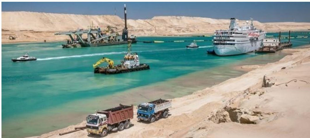
Figure 5-29 A satellite image of different dredging equipment for the Challenge Consortium at the work site (upper image) and picture of vessels (lower image)
