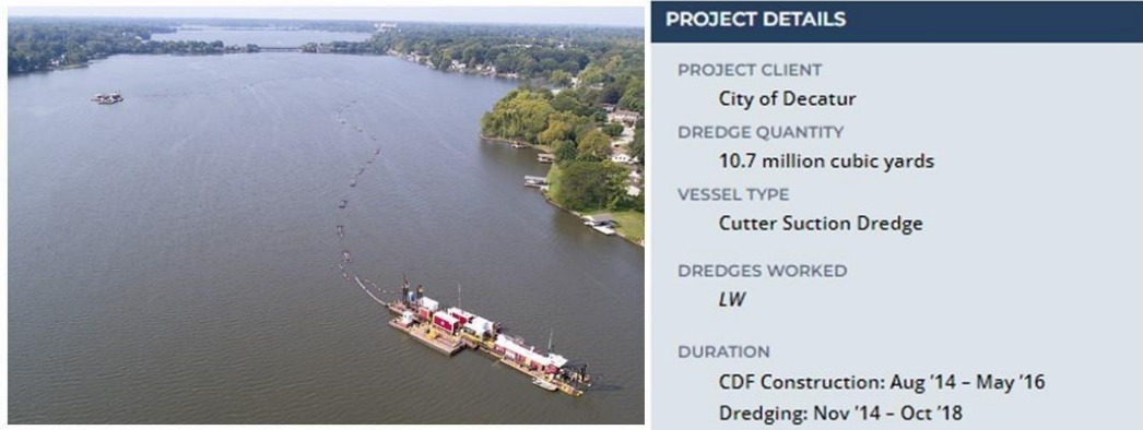
Figure 5-24 Lake Decatur (left) and the project details (Great Lakes Dredge & Dock Company)
